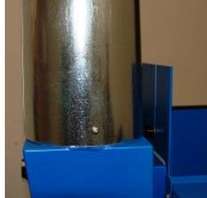
Figure 2. Exhaust Ventilation Stack
